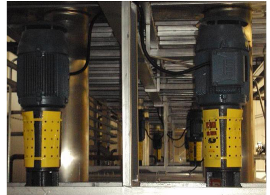
2 of the 12 Gusher 7550 Series pumps at the new AO Smith factory in Nanjing
