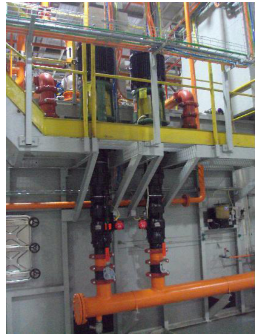
2 of the 6 PSI turbine pumps installed at the new Ford Transmission plant in Chong Qing.
