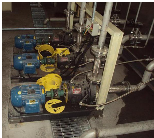
These 7071 Gusher Ansi Series pumps are part of the 6 now operating at the Nanjing location.
