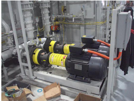
Shown here are 2 of 6 Gusher 7071 Series pumps now in use at the new Ford Engine Factory in Chong Qing.
