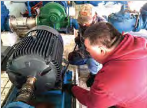
Great Southern service techs installing, calibrating and aligning a pump and motor.
