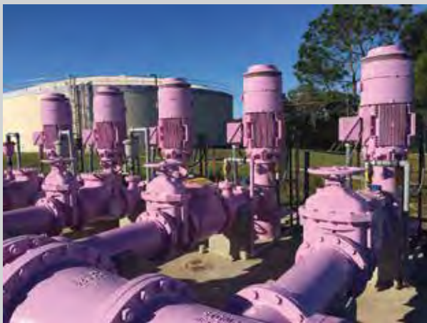
This installation includes five Deming® Vertical Turbine Pumps operating at 1250 GPM @ 278' TDH. These pumps are pumping reclaimed water.
