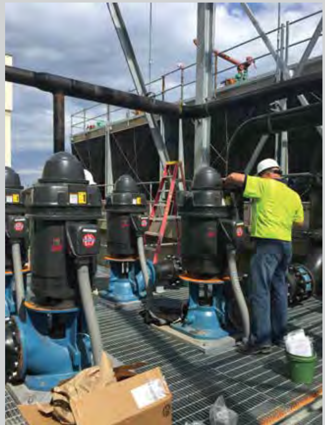
"Service After Sale"...a Great Lakes technician services this turbine installation, setting and calibrating impellers for system start up.
