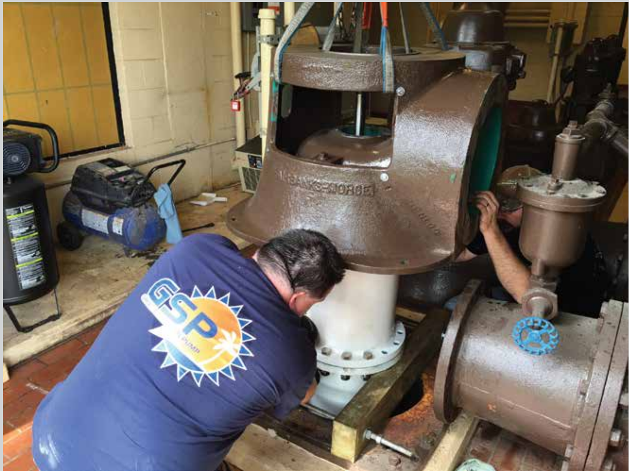
Great Southern technicians closing in on finishing a challenging Deming® Vertical Turbine Pump installation.
